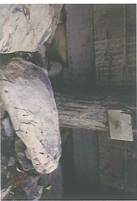
Figure 1-22: Minor undermining of the woods end abutment ballast wall.
