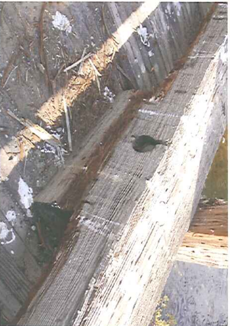
Figure 1-11: Typical rub damage on curb rail, rot initiated.
