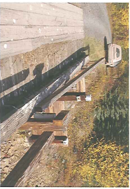
Figure 1-12: Broken rail at camp end downstream corner.
