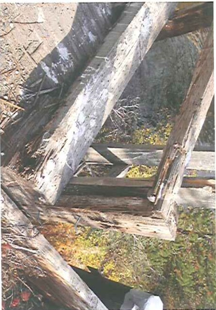
Figure 1-13: Damaged rail at woods end downstream corner.
