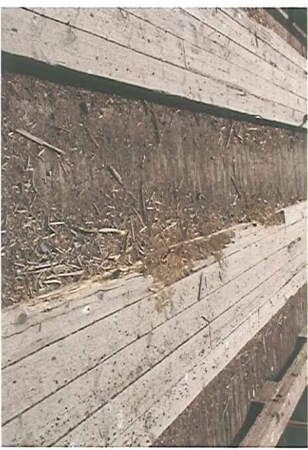
Figure 1-8: Rotten wearing deck plank.
