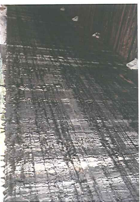
Figure 1-16: Typical unweathered face of girder.
